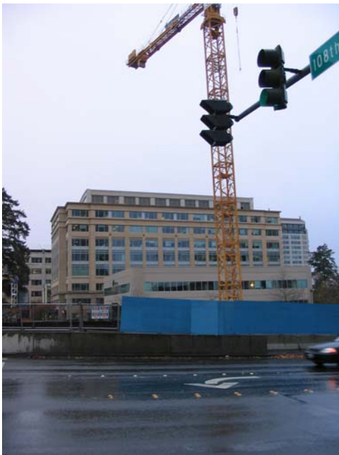
Figure 12. Original Tower Crane 4 Days Prior To Collapse
