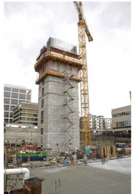
Figure 13. Replacement Tower Crane, Post Collapse
